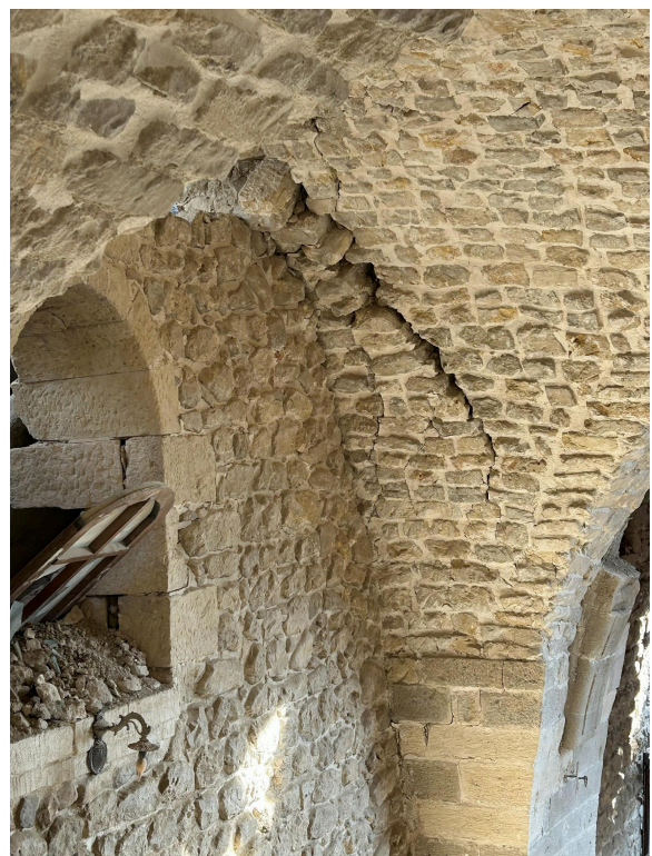
Fig. 12: Cracks on the northern wall
