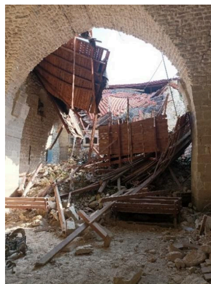
Fig. 2: Interior roof collapse
