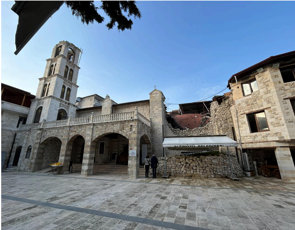
Fig. 4: External view of Saint Georgios Church, showing the destruction caused by the earthquake on the south wall and belltower
