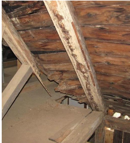
Support of beams and floors on different rooms. Roof structural problems.
